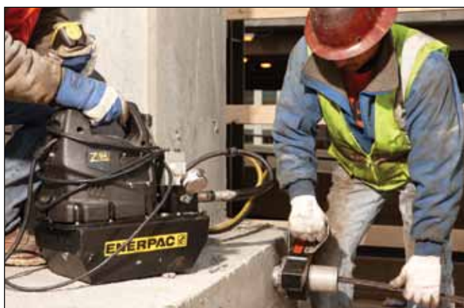
◀ The hydraulic PocketShear® makes quick and easy work of shearing tails on this elevated slab.
