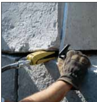
◀ A WR-5 wedgie cylinder is used to position a concrete block on a construction site.
