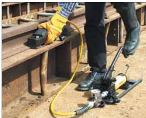
◀ Easily removing rusty nuts during railroad construction is just one of many application examples for the Enerpac Nut Cutters.
