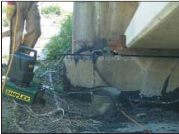
Simplex 70 Series pump & 50 ton flat jack cylinders makes easy work of bridge lifting. "We had to make complete bearing change outs on 90 bridges along Interstate 80. The Simplex 70 Series pump with its permanent magnet motor just kept running even with long extension cord and portable generator power."
